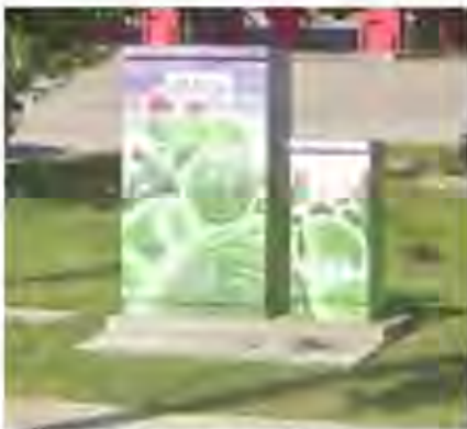
Traffic signal box – Woodstock, VA Image capture: Aug 2022 © 2022 Google
